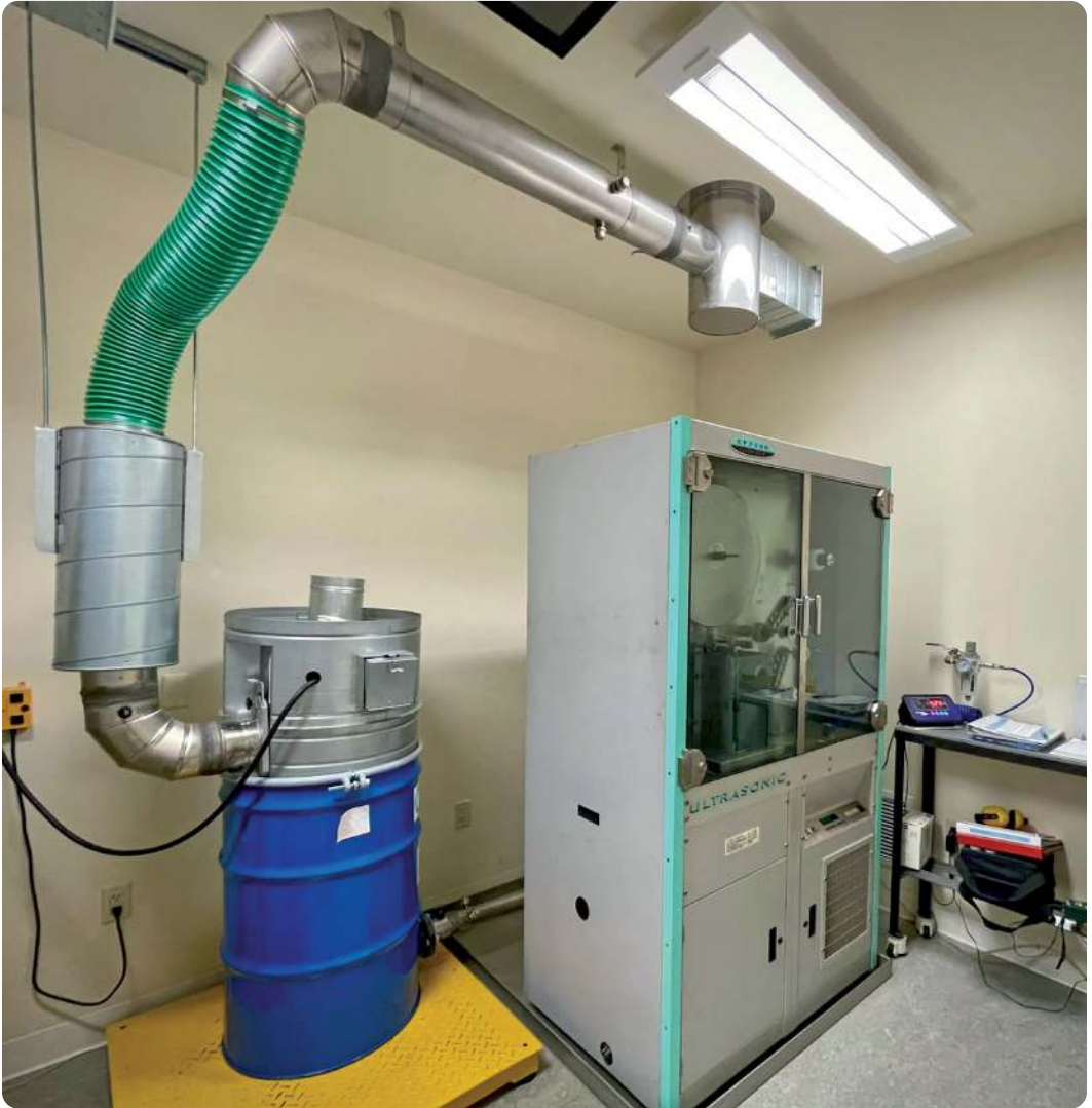
Figure 5. PHI carbon capture system.
